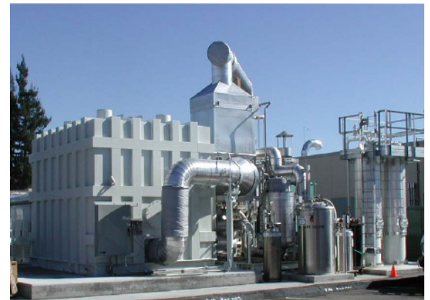
FuelCell Energy 1.4 MW system
