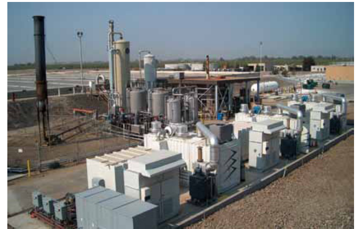
FuelCell Energy 1.2 MW system
