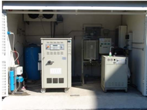
Electrolyser and purification stage for continuous hydrogen production
