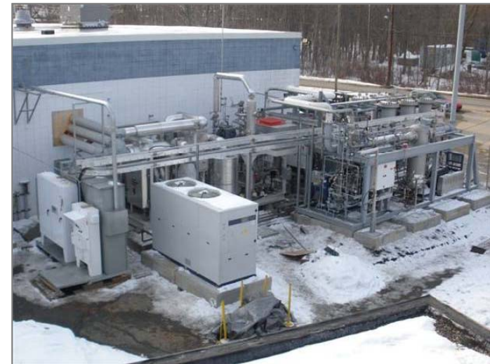
Anode Exhaust Processing and H 2 PSA
